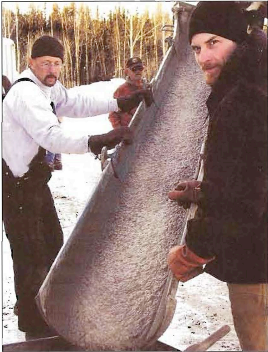
Jack Herbert, left, and Xavier Schlee direct cold-weather concrete to the pour site adjacent to the CCHRC facility in Fairbanks.
